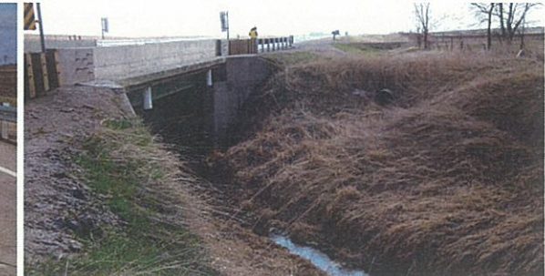
Stream bank on south side of bridge
