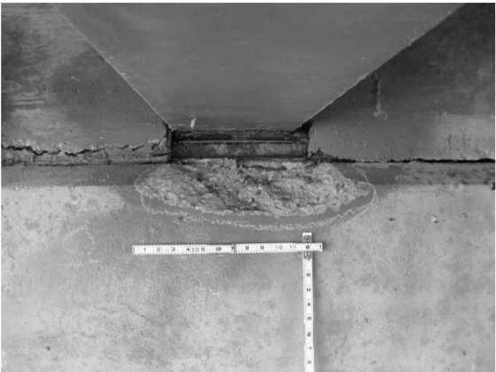
Deterioration of far- left abutment
