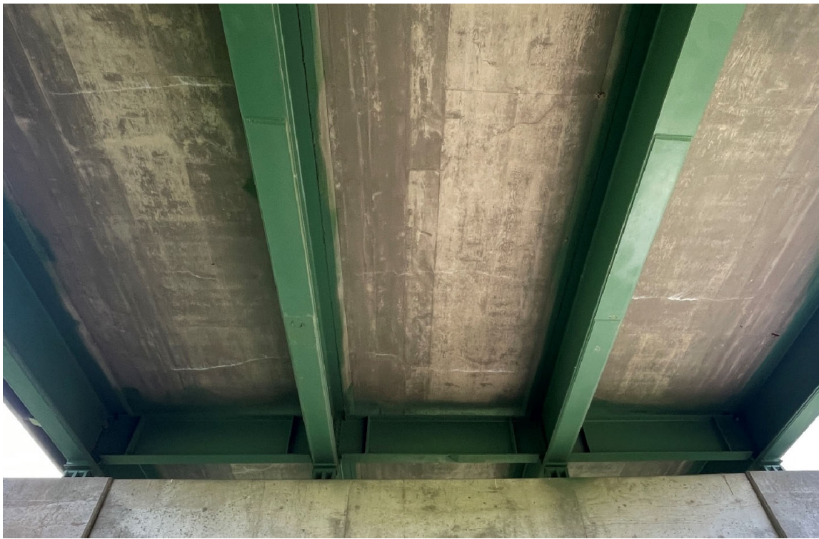
Image 21: Deck Cracking, Typ.
