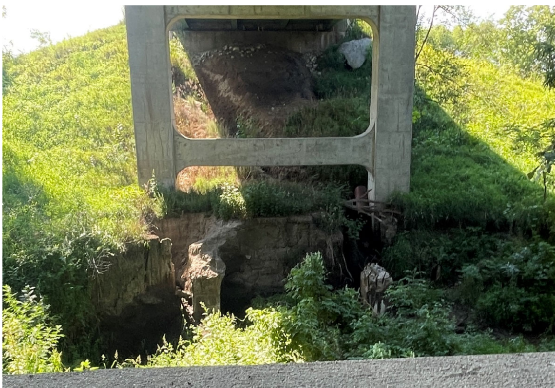
Image 20: Near Berm Erosion (Looking West)
