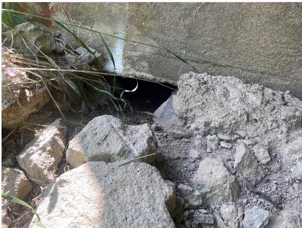
Image 12: Near Abutment Undermining (South Side)
