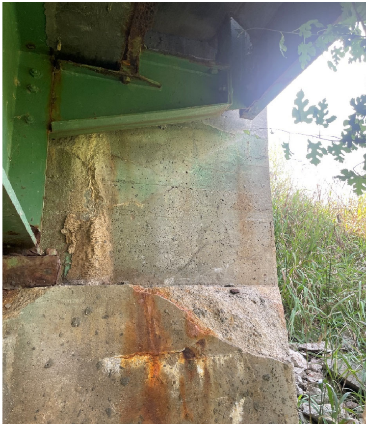
Image 17: Near Abutment Spalling (North Side)
