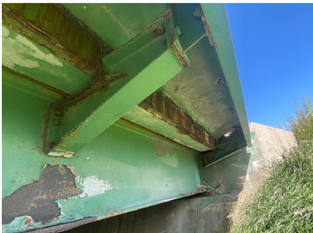
Image 26: Exterior Girder Rusting (South Side)
