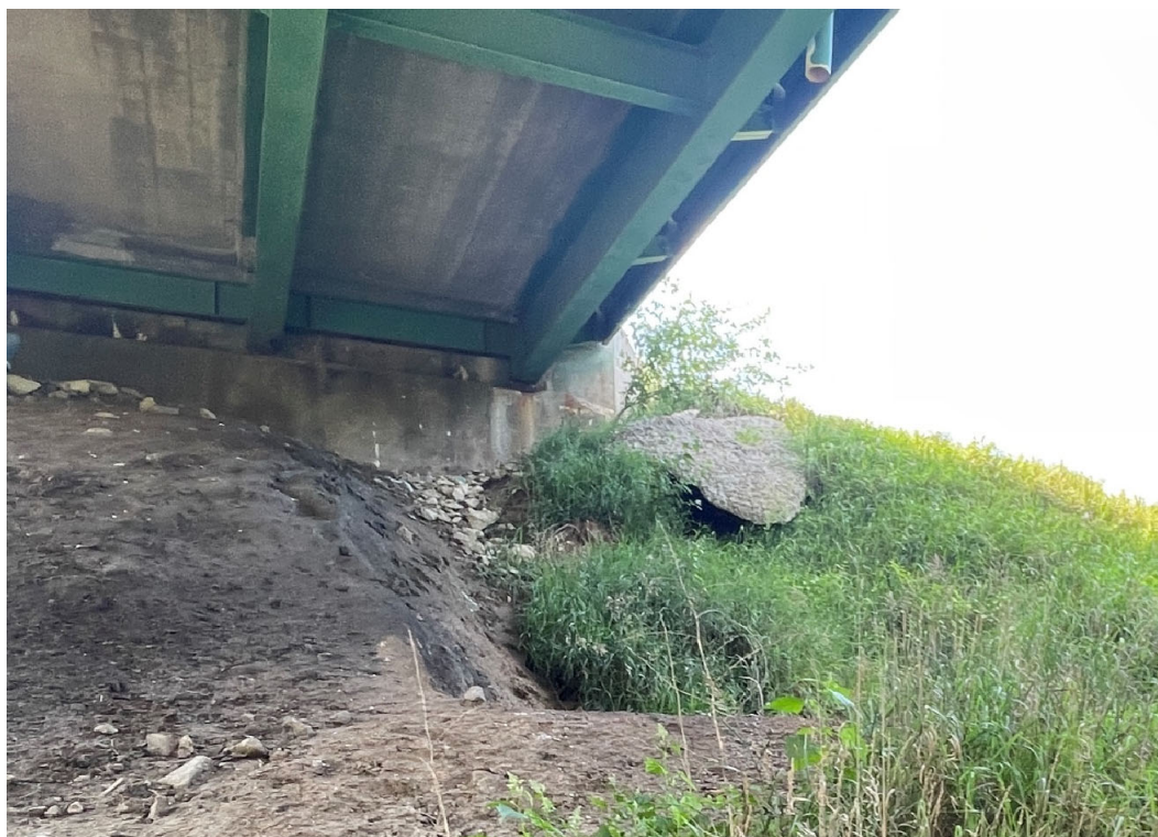
Image 14: Near Berm Erosion (North Side)
