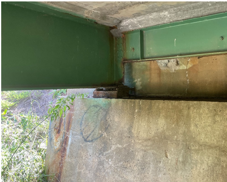
Image 8: Near Abutment Spalling (Looking Northwest)
