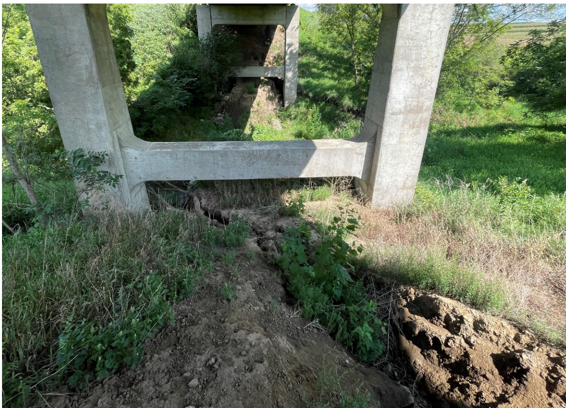
Image 19: Near Berm Erosion (Looking East)
