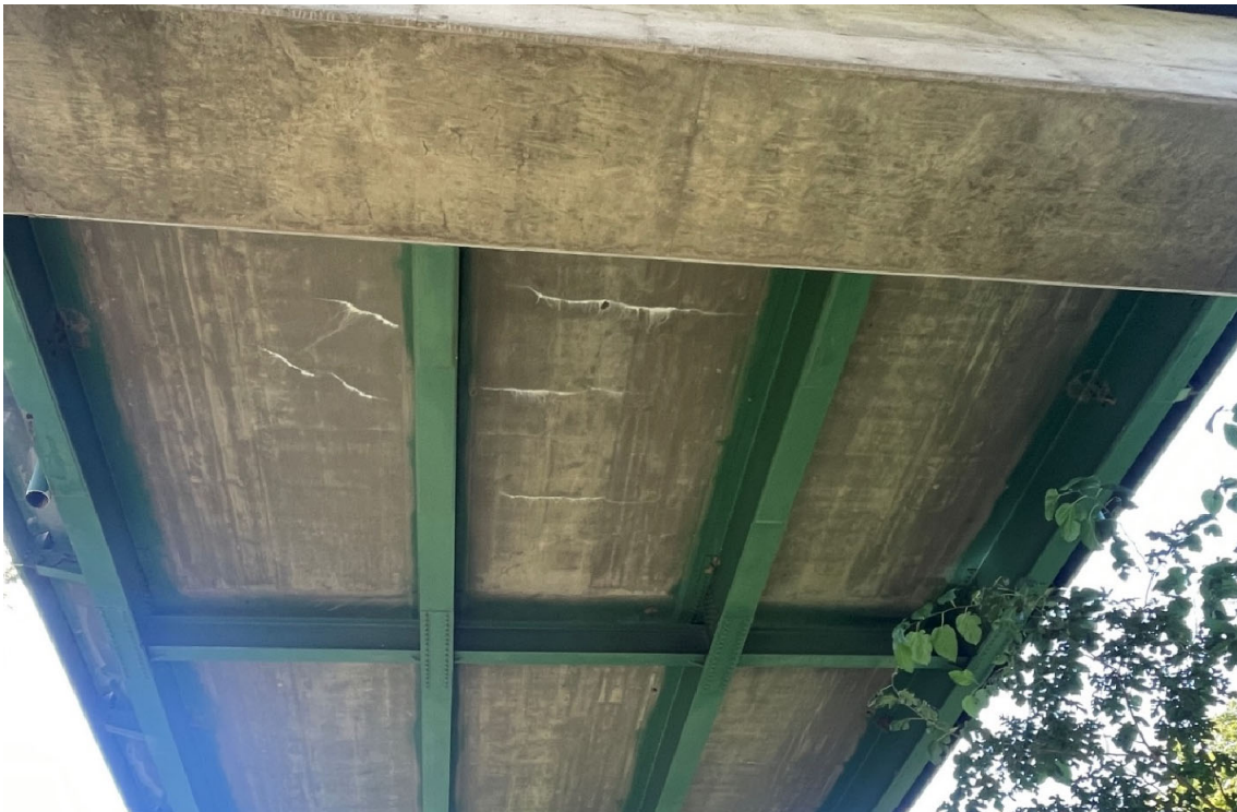
Image 28: Deck Cracking in Middle Span, Typ.
