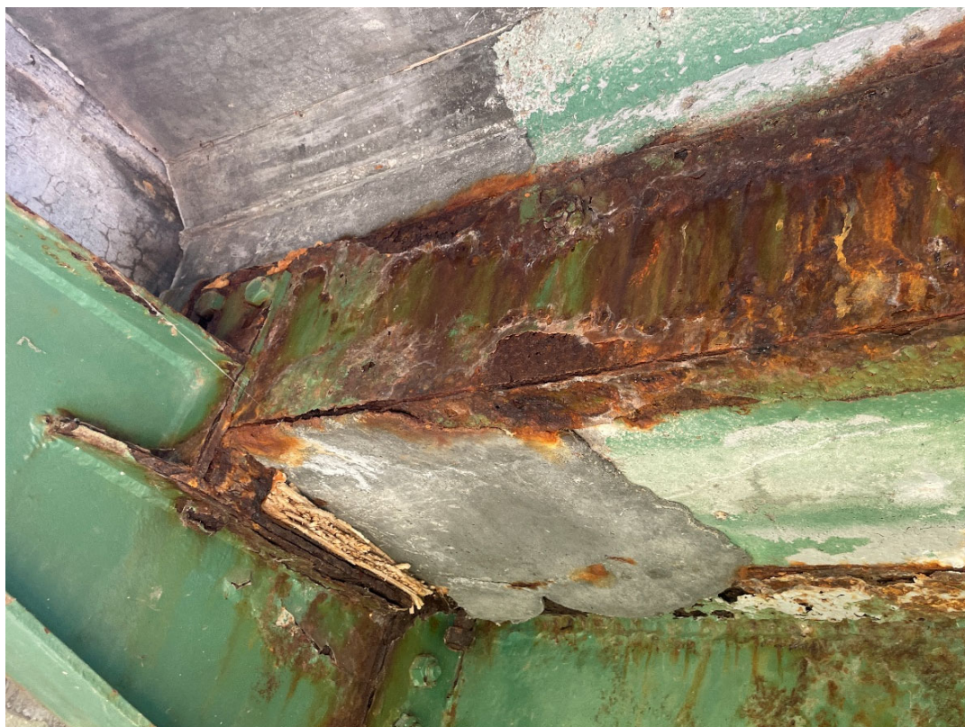
Image 10: Section Loss at Near Abutment Exterior Girder
