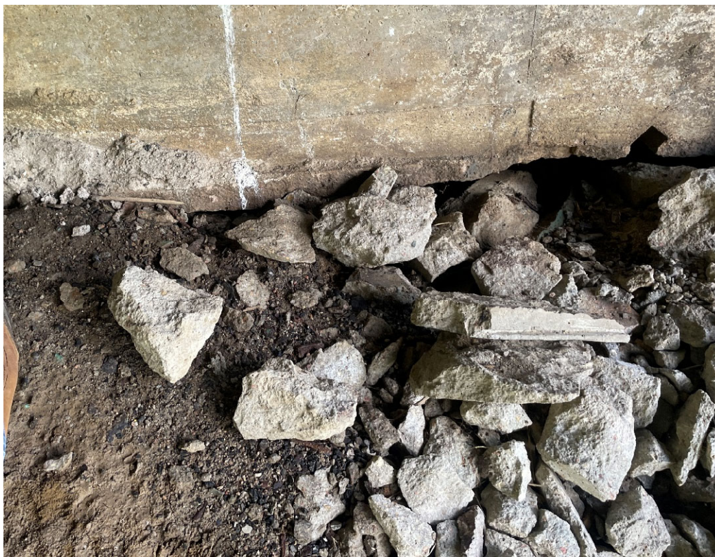
Image 15: Near Abutment Undermining (North Side)
