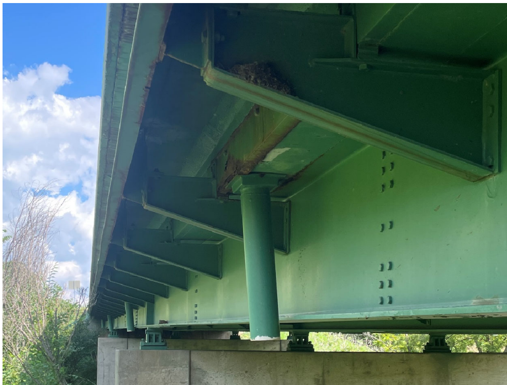
Image 18: Drain Leakage (North Side)
