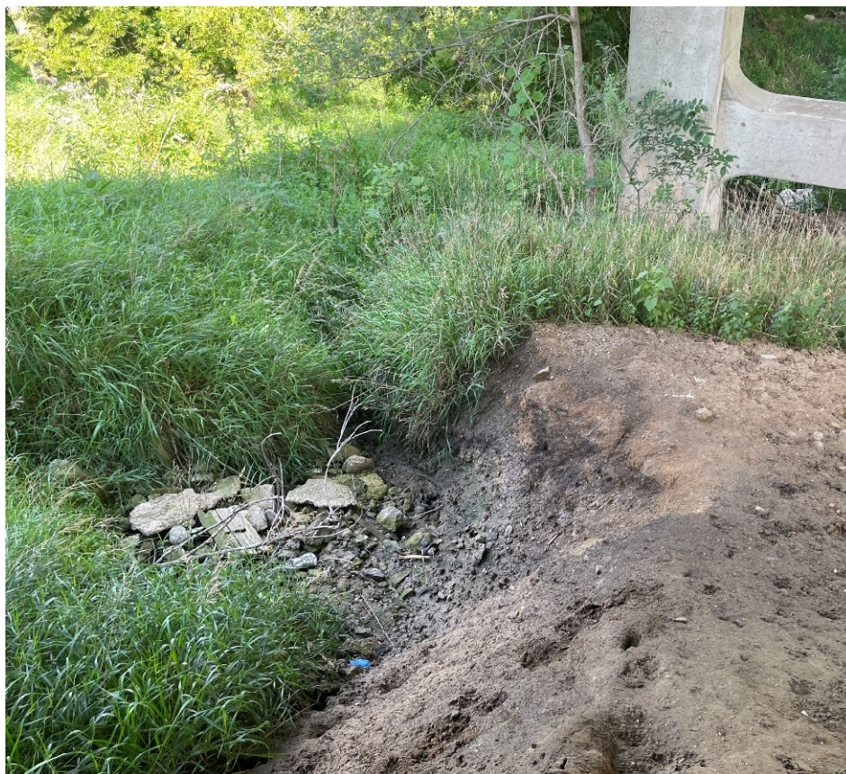
Image 13: Near Berm Erosion below Drain (North Side)
