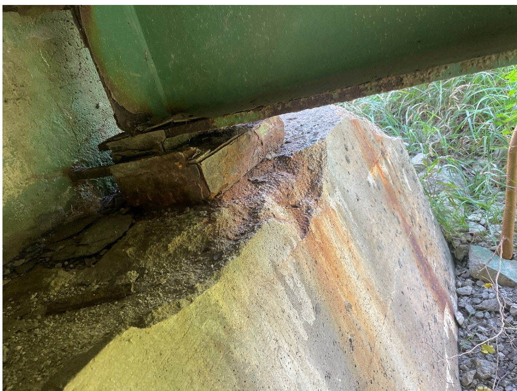
Image 16: Near Abutment Spalling (North Side)
