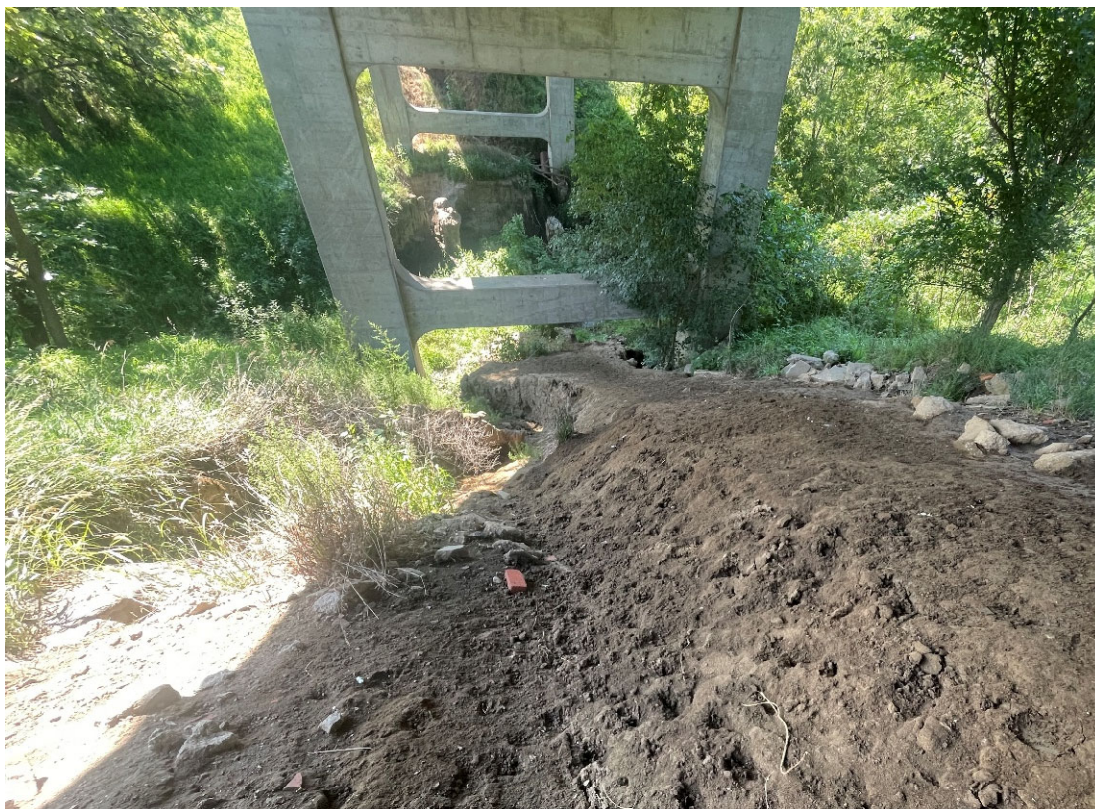
Image 25: Far Berm Erosion (Looking West)
