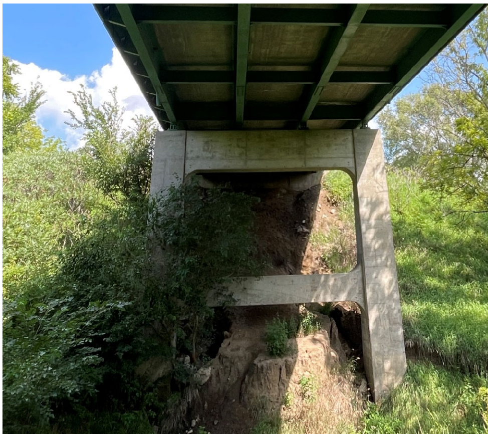
Image 22: Far Berm Erosion (Looking East)
