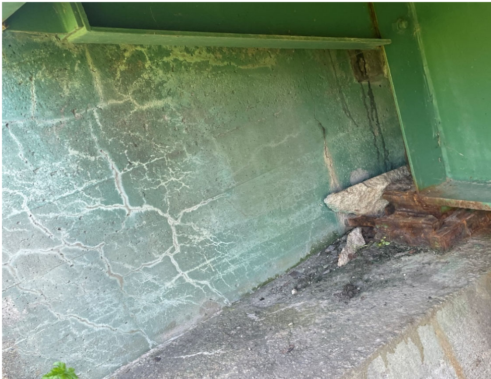
Image 24: Far Abutment Cracking (Looking East)
