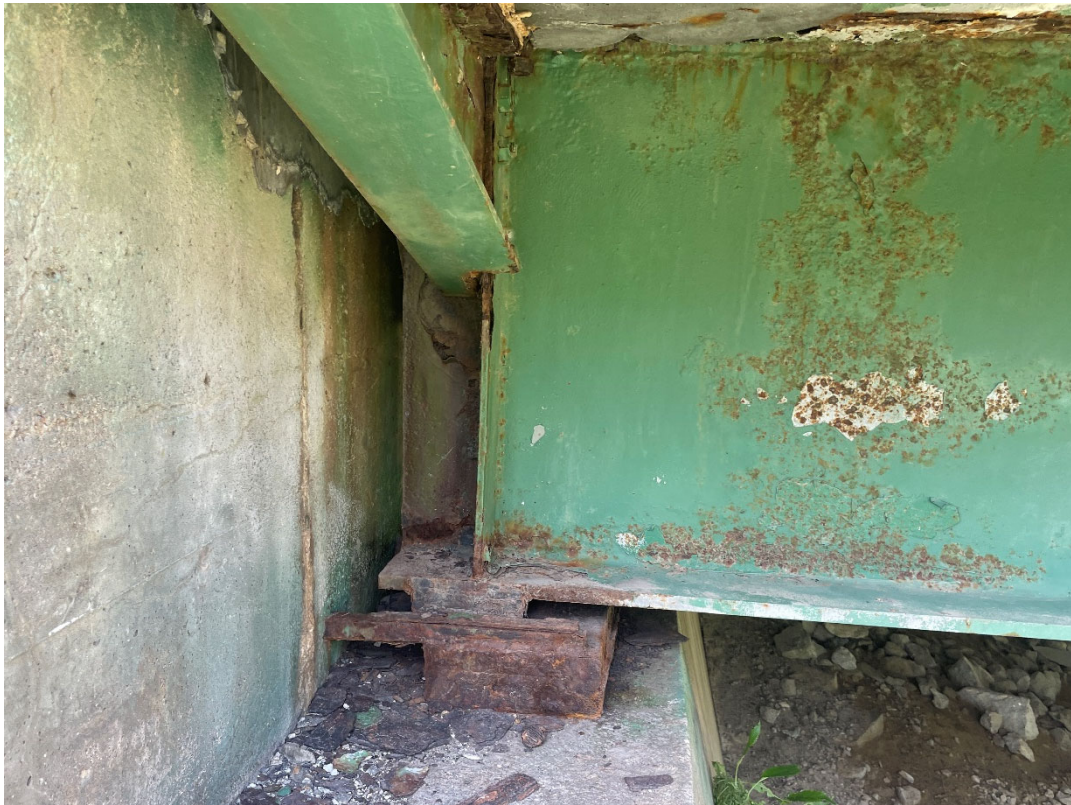
Image 9: Near Abutment Bearing Rusting, Typ.
