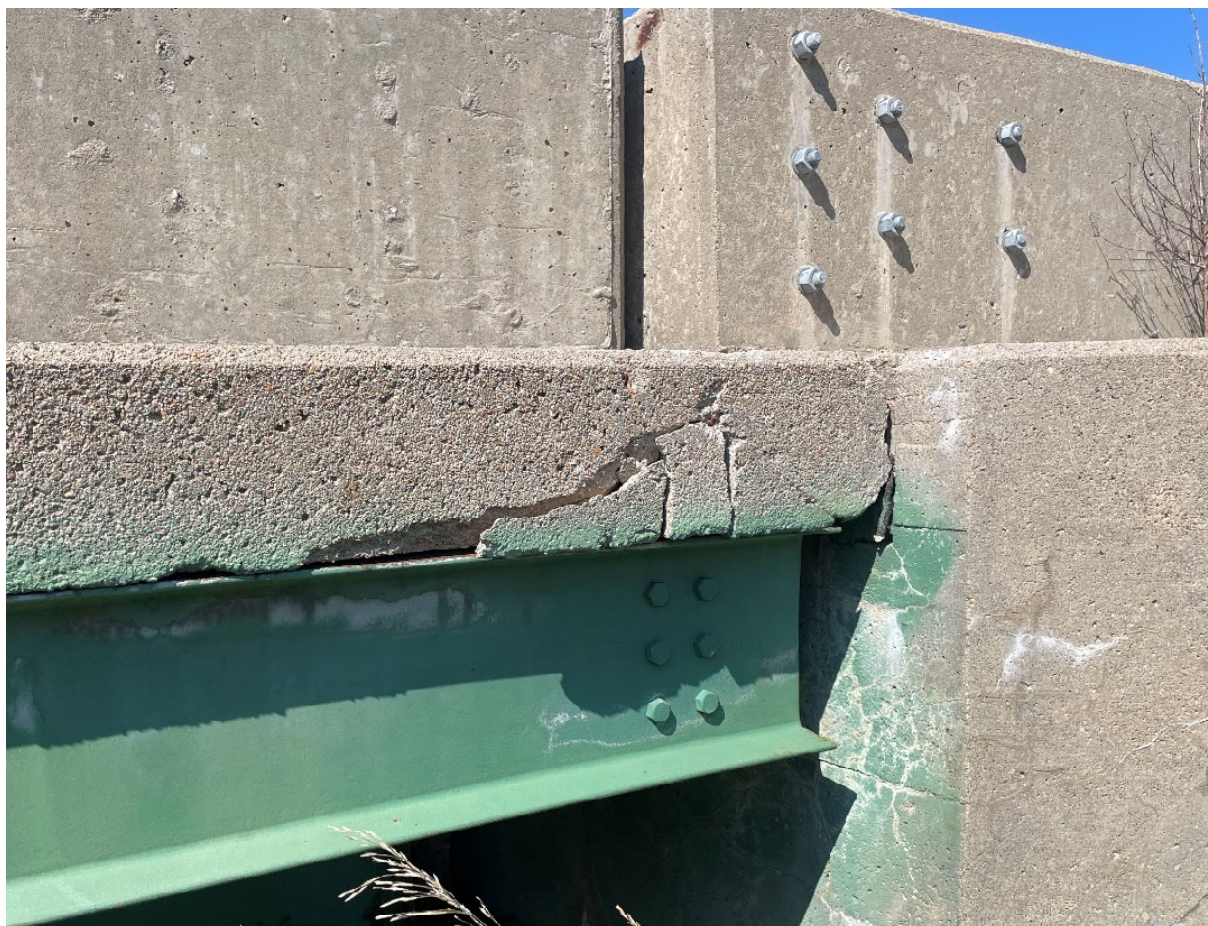
Image 29: Deck Edge Spalling (South Side)
