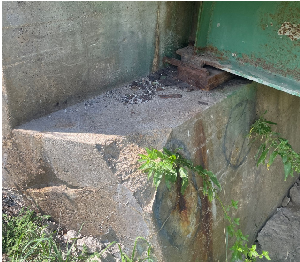
Image 7: Near Abutment Spalling (South Side)
