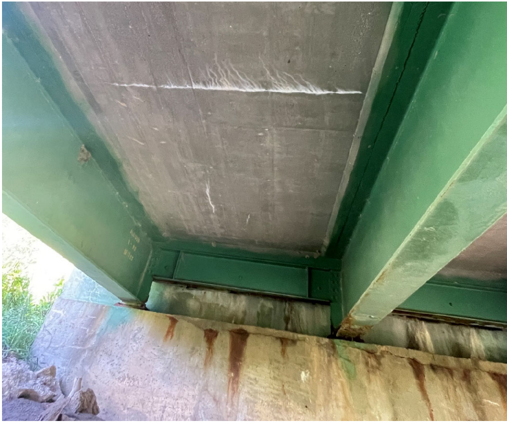
Image 27: Deck Cracking (South Side)
