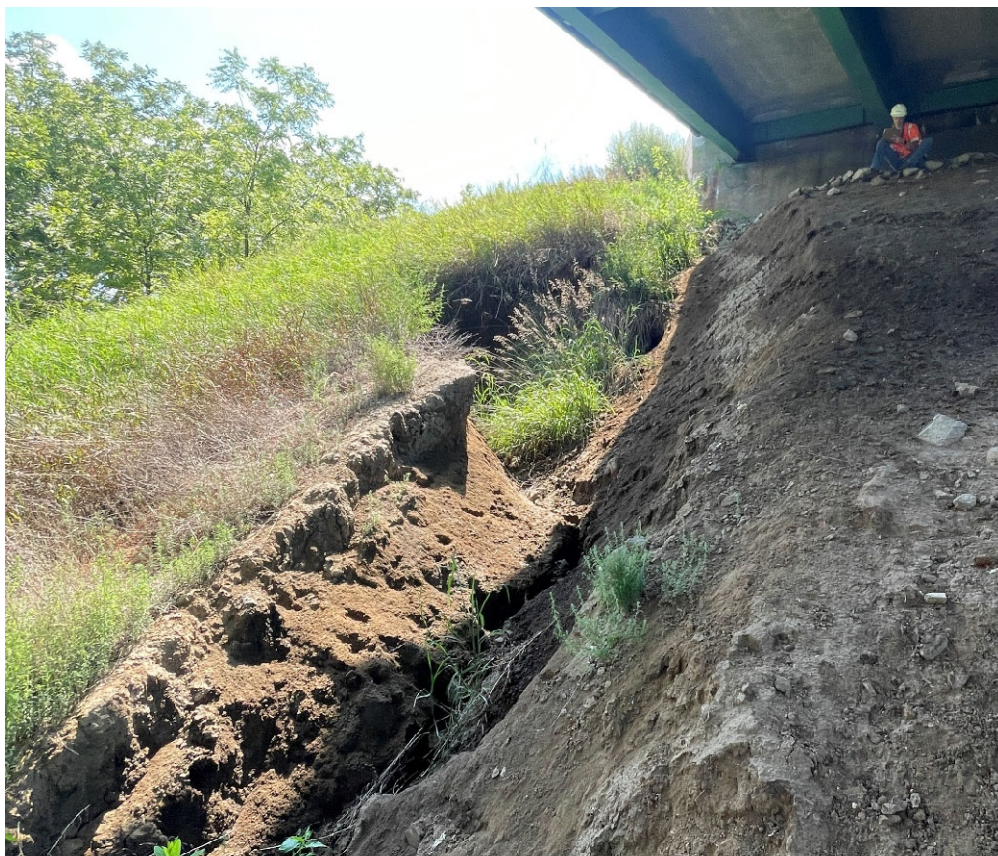
Image 11: Near Berm Erosion (South Side)
