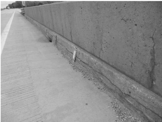
Barrier rail deterioration
