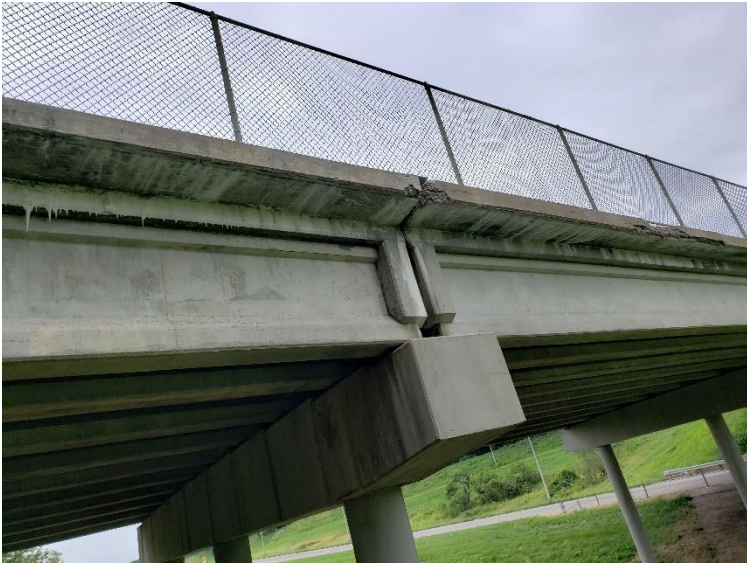
Deterioration of west overhang at pier 3
