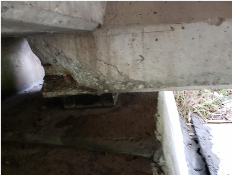
Spalled beam end at north abutment
