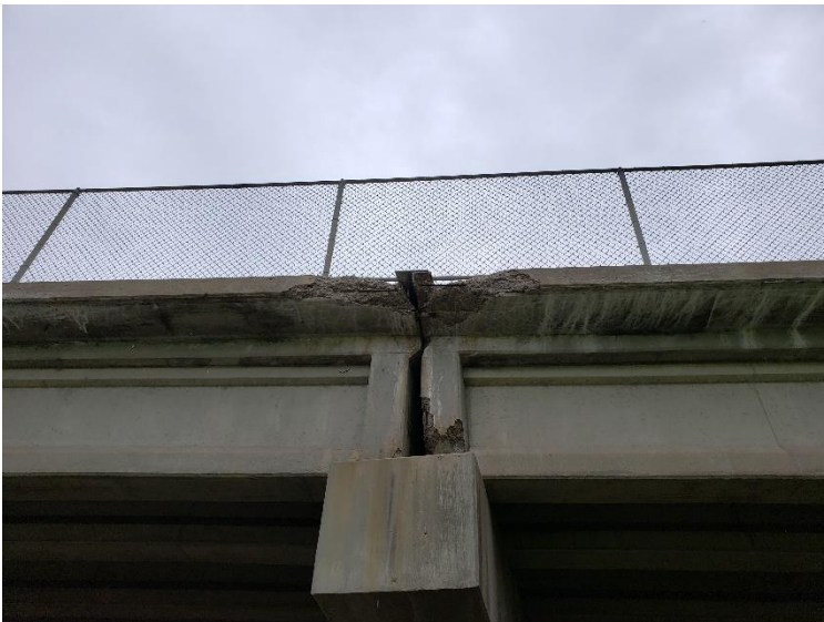
Deterioration of west overhang at pier 1
