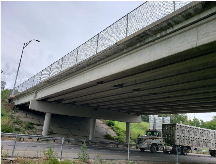
Leaching and spalling on west overhang
