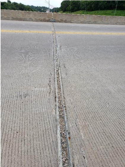
Cracking along pier joint
