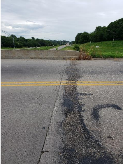
Deterioration at south end of bridge
