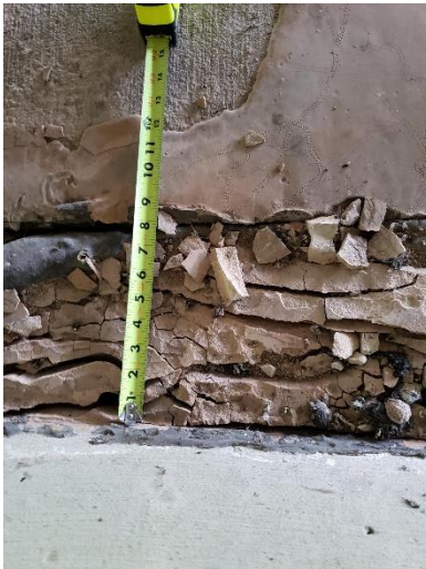
Gap at top of slope protection
