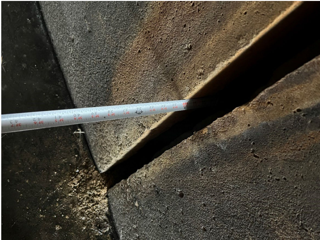
Void at Center Construction Joint of South Barrel
