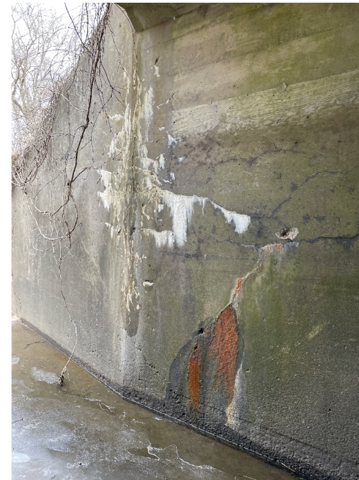
Typical Delamination (Northwest Wing Shown)
