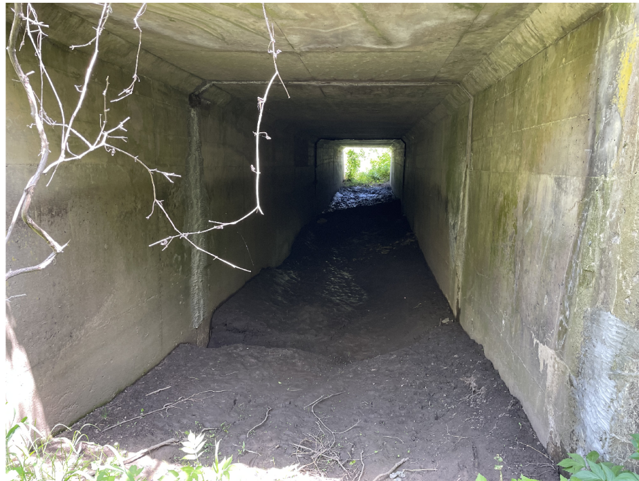
Sediment Buildup (South Culvert Barrel)
