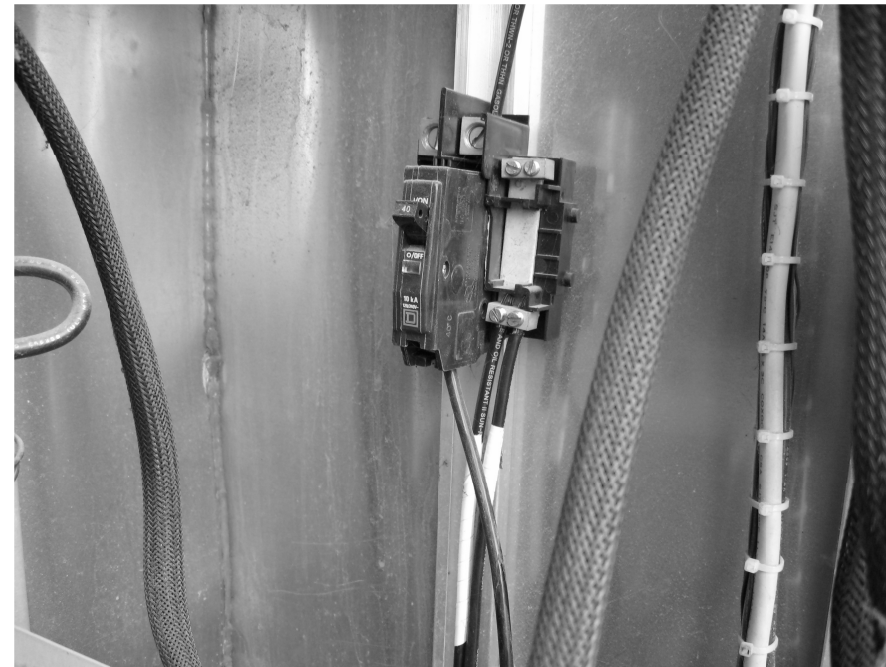
TYPICAL BREAKER INSTALLATION IN SIGNAL/CONTROLLER CABINET
