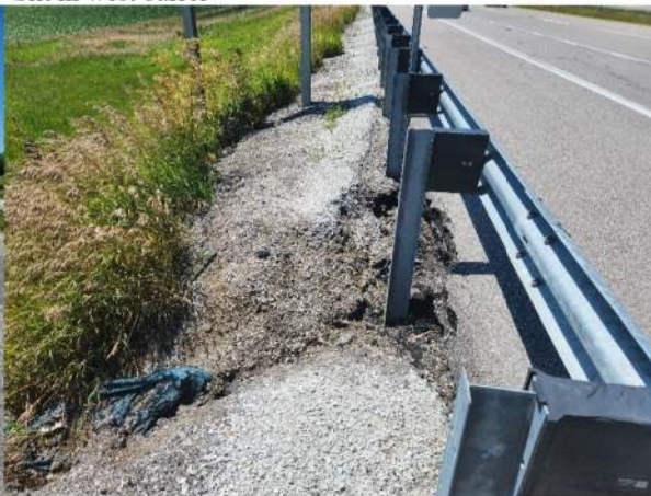
Erosion/undermining at shoulder behind south guardrail
