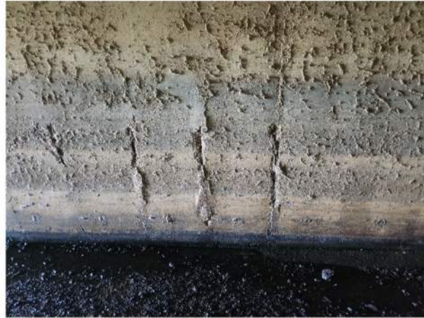
Shallow bars exposed in wall
