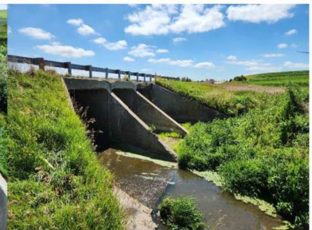
North headwall (silt/vegetation center and west)
