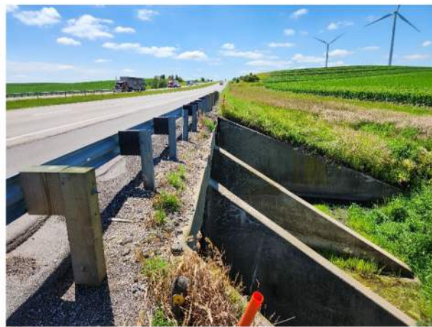
Damaged post/missing spacer block at N guardrail
