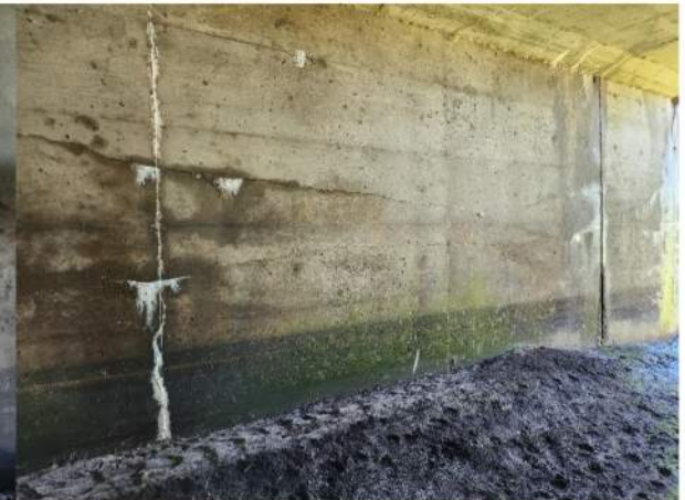
Typical exterior wall (horiz. leaking cracks)
