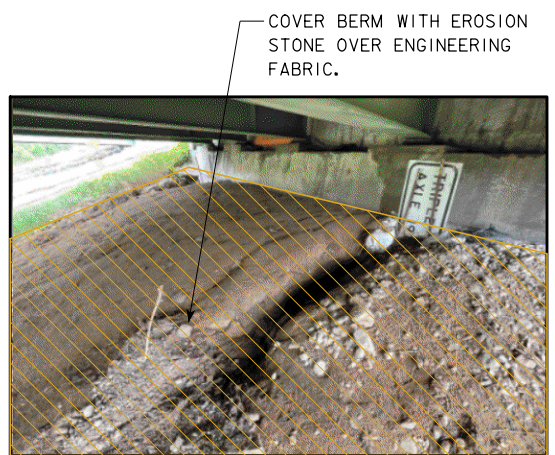
BERM EROSION AT EAST ABUTMENT
