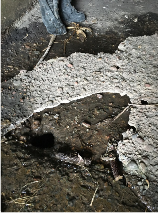
Holes in the floor of the box.
