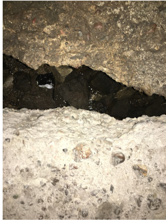
Crack across the entire floor near the downstream end. Water also running under the concrete floor.
