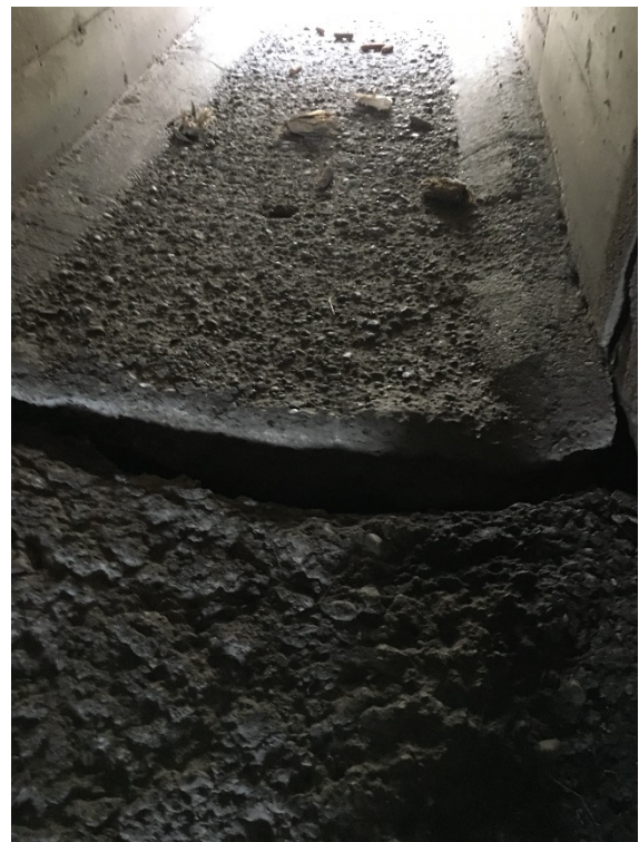
Crack across entire floor near outlet end
