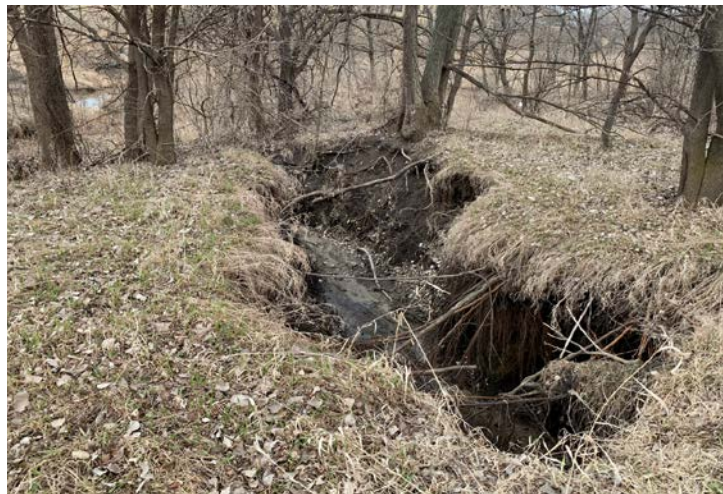
3. Erosion on north side of letdown
