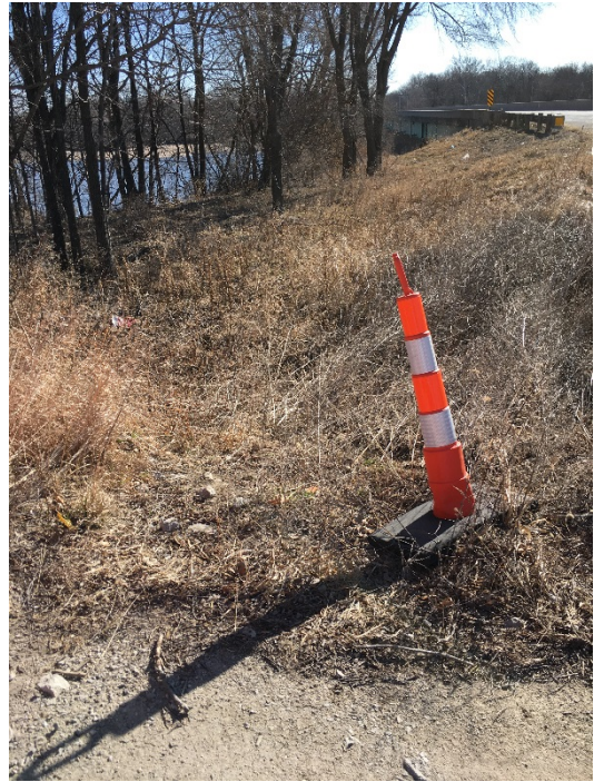
Channelizer on the east side of the entrance denoting the sinkhole
