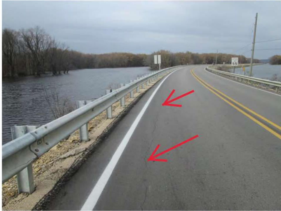
Attachment 1 – Longitudinal cracking in 2019 resurfaced pavement
