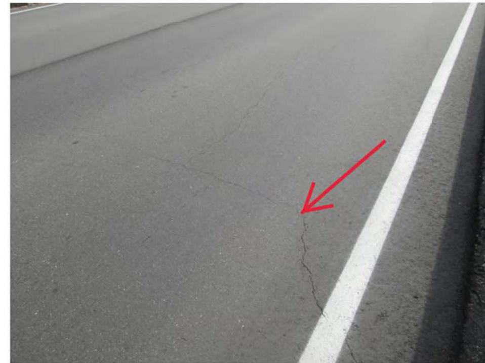
Attachment 1 - Cracking in 2019 resurfaced pavement
