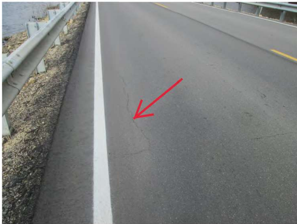
Attachment 1 – Cracking in 2019 resurfaced pavement
