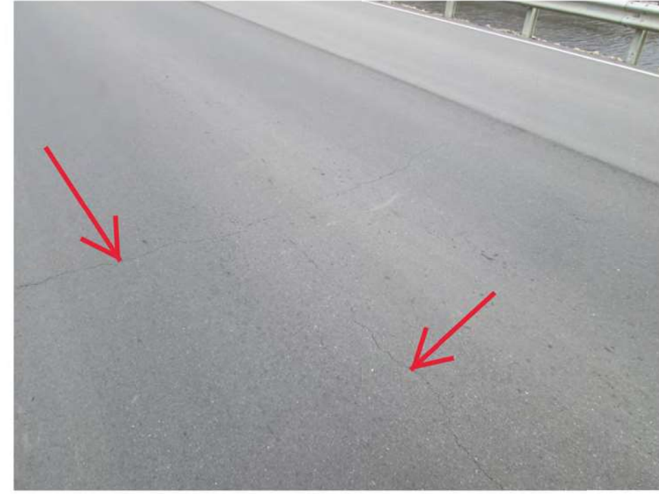
Attachment 1 - Cracking in 2019 resurfaced pavement
