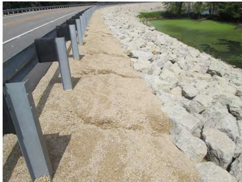
Attachment 1 – Shoulder erosion at new shoulder
