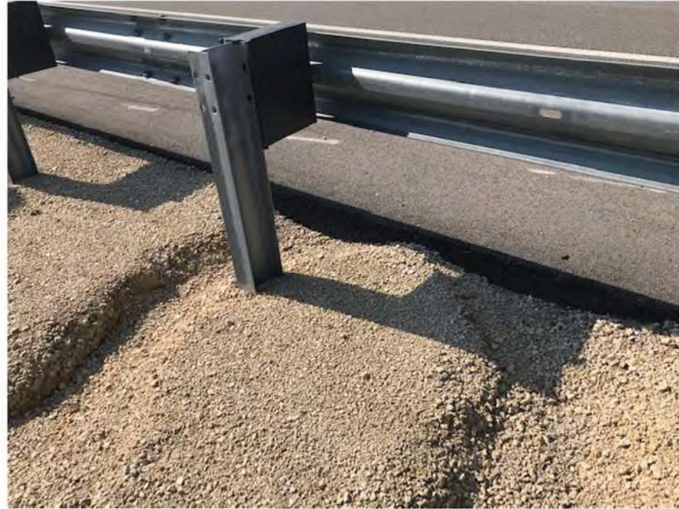
Attachment 1 – Close up of erosion at shoulder
