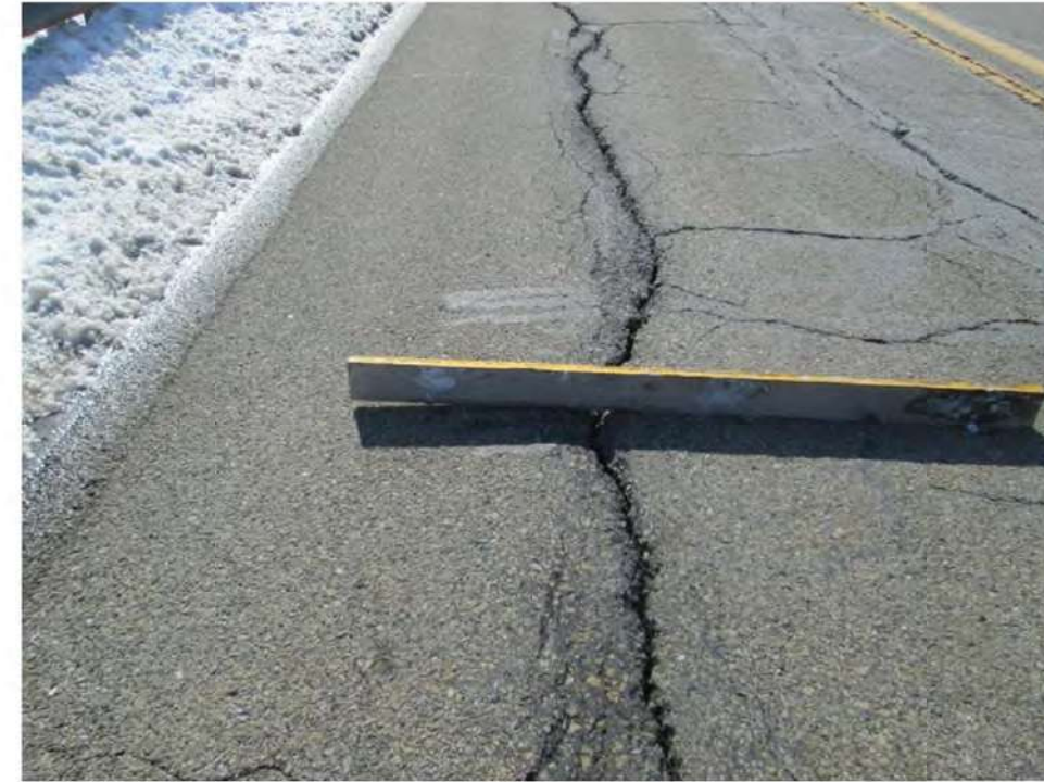
Attachment 1 – Previously existing Pavement Cracking Eastbound prior to 2019 resurfacing
