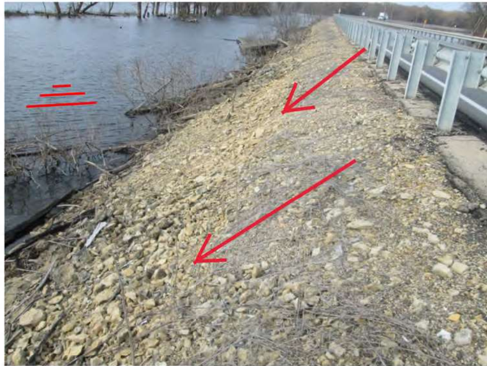
Attachment 1 – wave action/current and rip-rap movement along fore-slope. Note: debris movement along face of embankment
