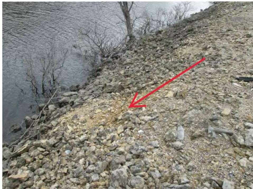
Attachment 1 – rip-rap movement/erosion along face of fore slope as shown in discolored area.
