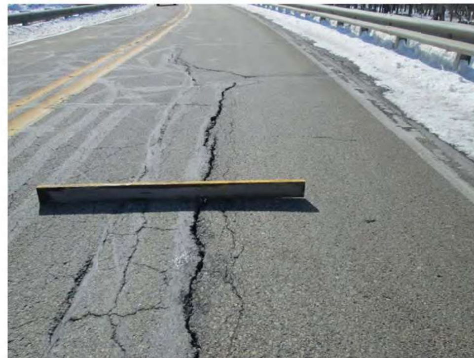
Attachment 1 – Previously existing Pavement Cracking Westbound prior to 2019 resurfacing
