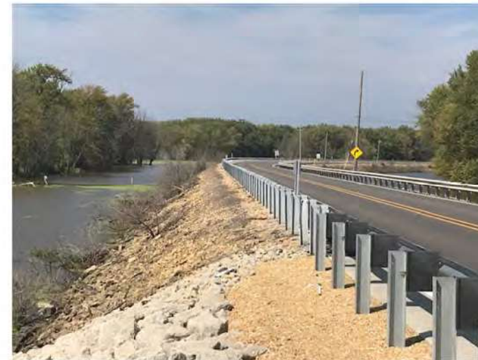
Attachment 1 – Looking north at transition from overflow bridge rip-rap to existing rip rap slope
