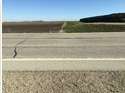
Damaged pavement about the pipe
