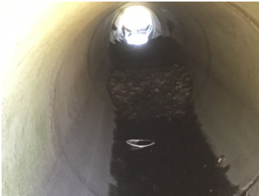
Dirt pile caused by pipe separation
